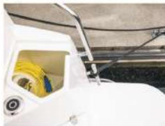
Protected connection for shore power.
